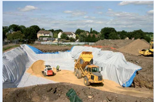
Stage 4: Protect the root barrier membrane from tyre damage with a layer of sand.
